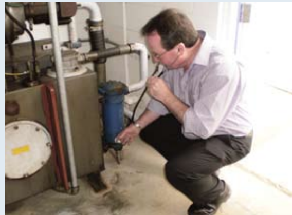
Warren Crighton, Bluff Assistant Manager, checking for a water leak
