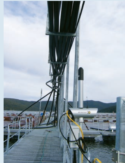
Surface camera (foreground) and overhead feed lines that supply each distributor
