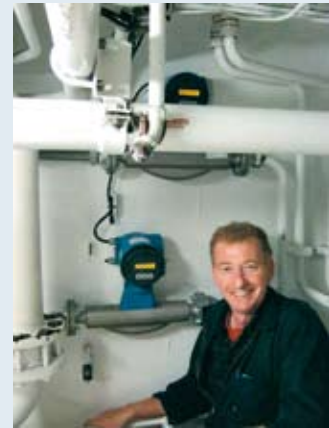
Peter Robertson, Chief Engineer, on the San Discovery with fuel meters installed on vessels to give more precise monitoring of fuel usage during trips
