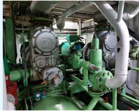
ABOVE The ammonia compressor, located in the refrigeration room, on board San Waitaki. 1
