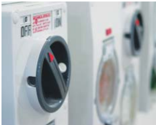
Sanford is a heavy user of electricity, mainly due to energy requirements of freezing and coldstorage; our total usage equals that of a small town
