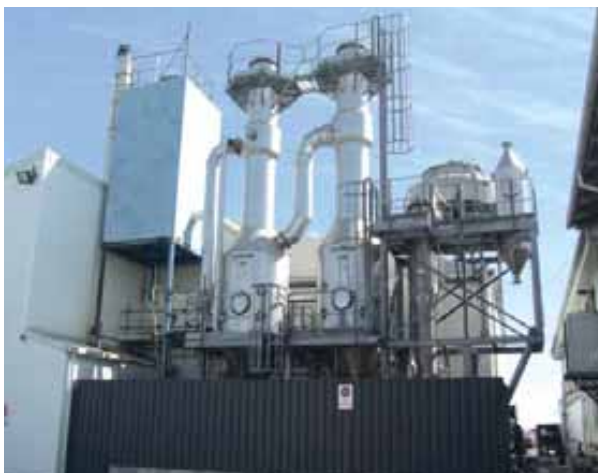
Fishmeal plant evaporator installed in Timaru.
