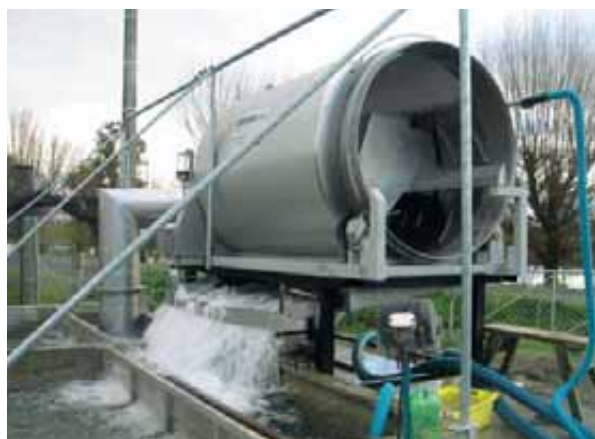
Screens installed to remove Didymo, Kaitangata hatchery.
